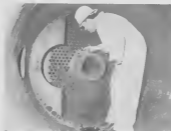
A. Tromp inspecting waste heat boiler at H2AR for corrosion and cleanliness prior to calling the Government boiler inspector.
